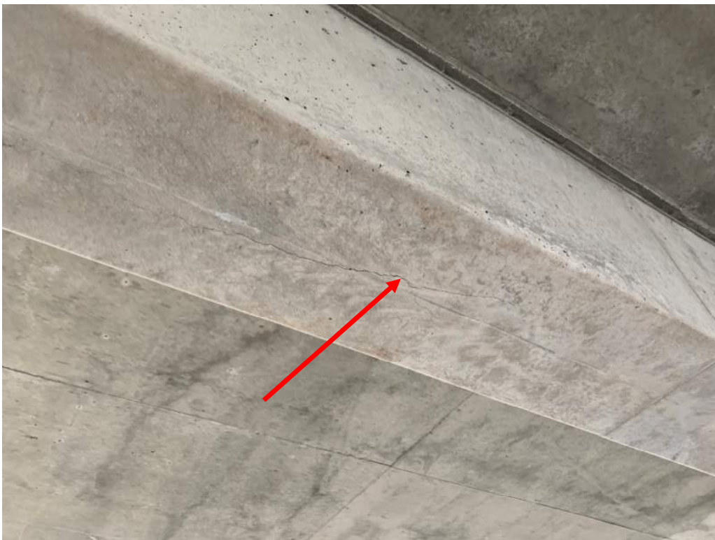
Photo 10 – Expansion Structure – Crack in bottom of beam supporting level 5 at grid C between grids 8 & 10 (Grid J similar)
