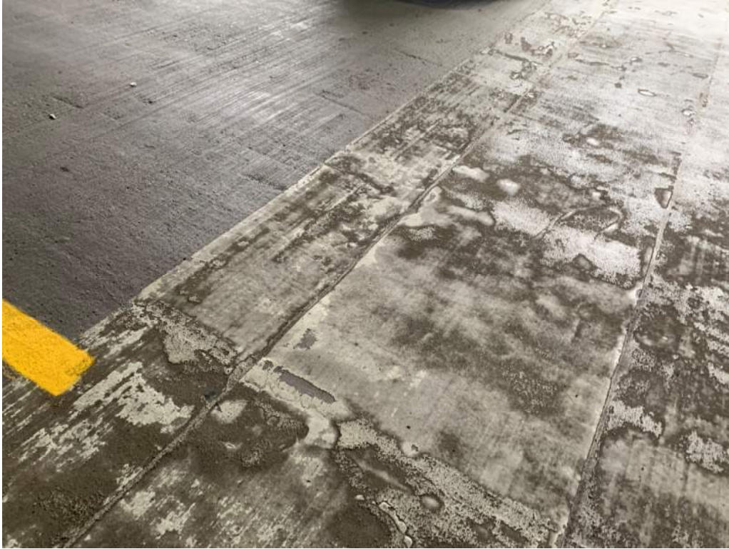
Photo 3 – Original Structure – Failed traffic coating over concrete pour strip (Level 3 shown, other levels similar)
