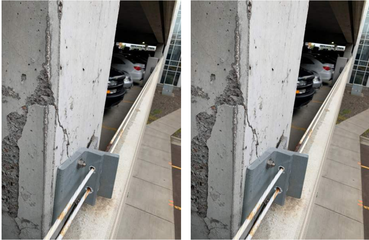
Photos 5 – Original Structure – Cracked and spalled column corner at N/5 (barrier strand anchorage) between levels 2 and 3.
