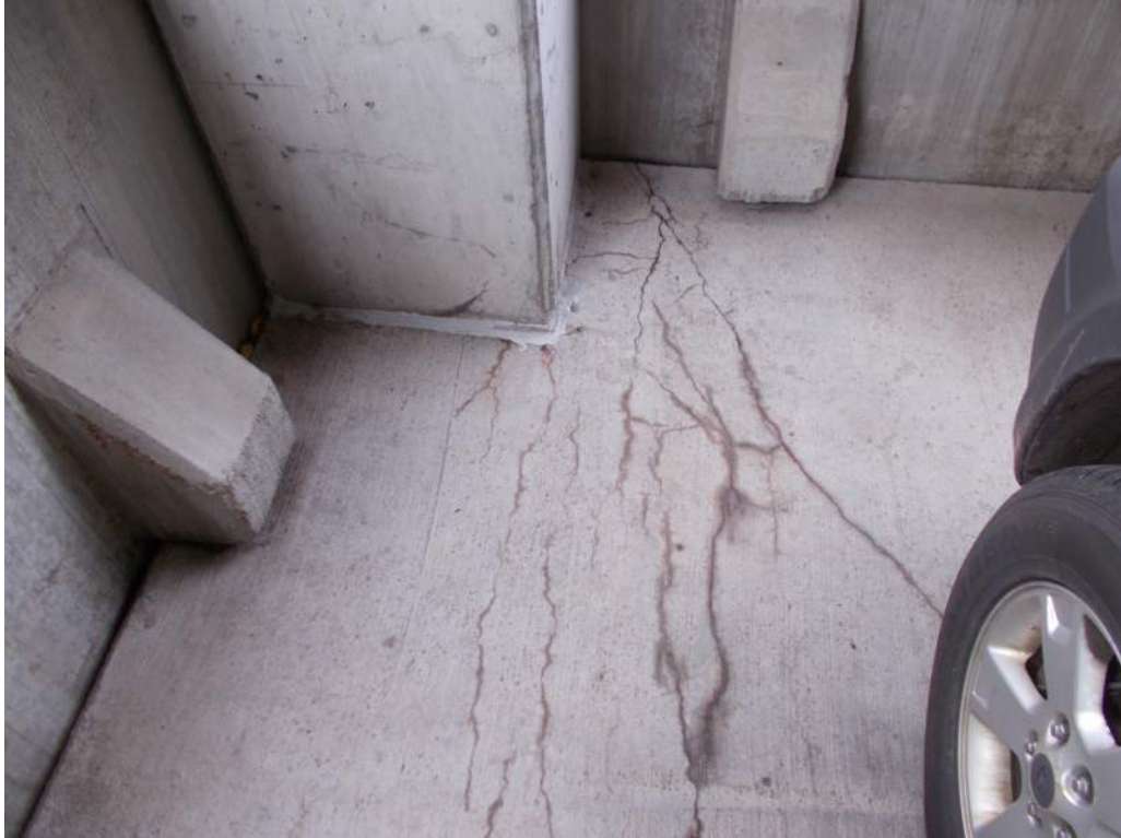
Photo 1 – Original Structure – Hairline cracking in elevated deck at column
