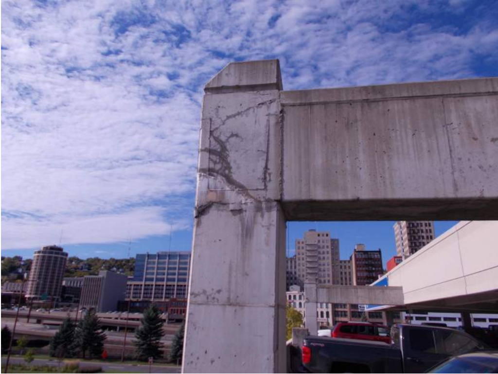
Photo 7 – Original Structure – Cracked top of column at Grid B/4 (B/3 similar)
