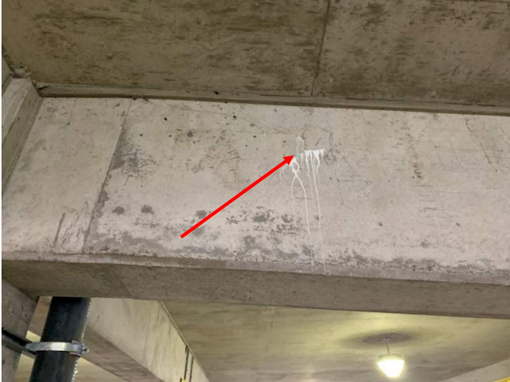
Photo 11 – Expansion Structure – Crack in beam web supporting level 5 on grid 8 between grids K & L
