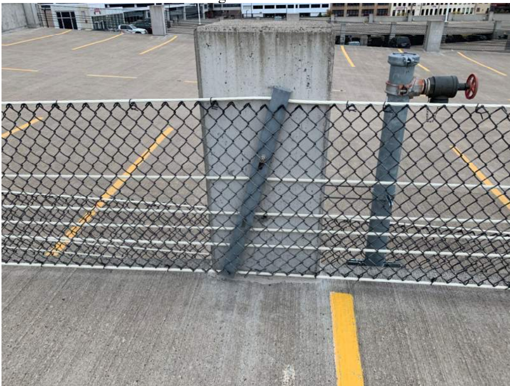
Photo 12 – Expansion Structure – Loose barrier cable bracket at column J/8
