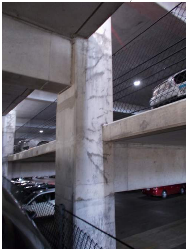
Photo 4 – Original Structure – Typical hairline column cracking at staggered beam interface
