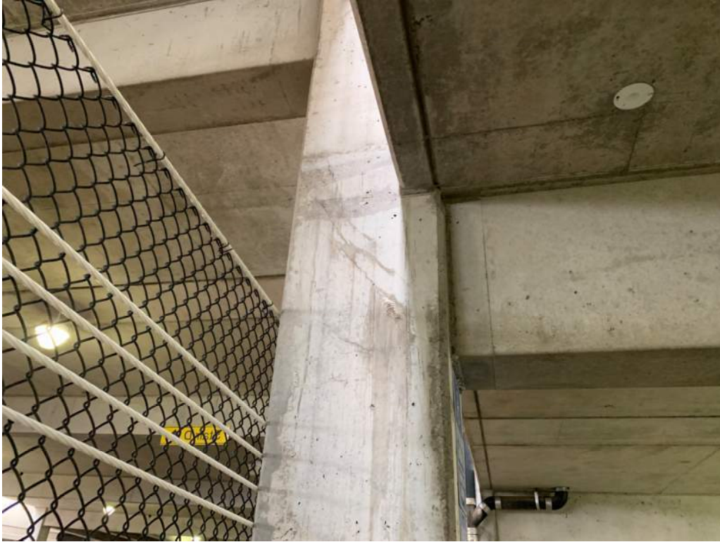
Photo 9 – Expansion Structure - Typical hairline column cracking at beam interface
