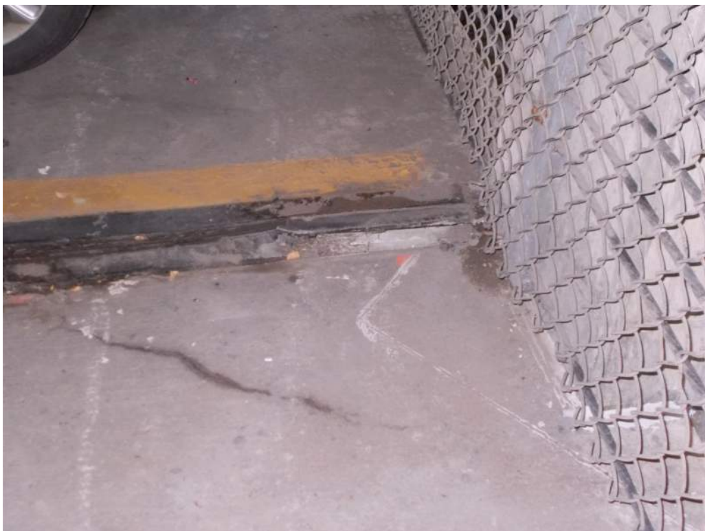
Photo 2 – Original Structure – Failed expansion joint at slab on grade to elevated slab interface
