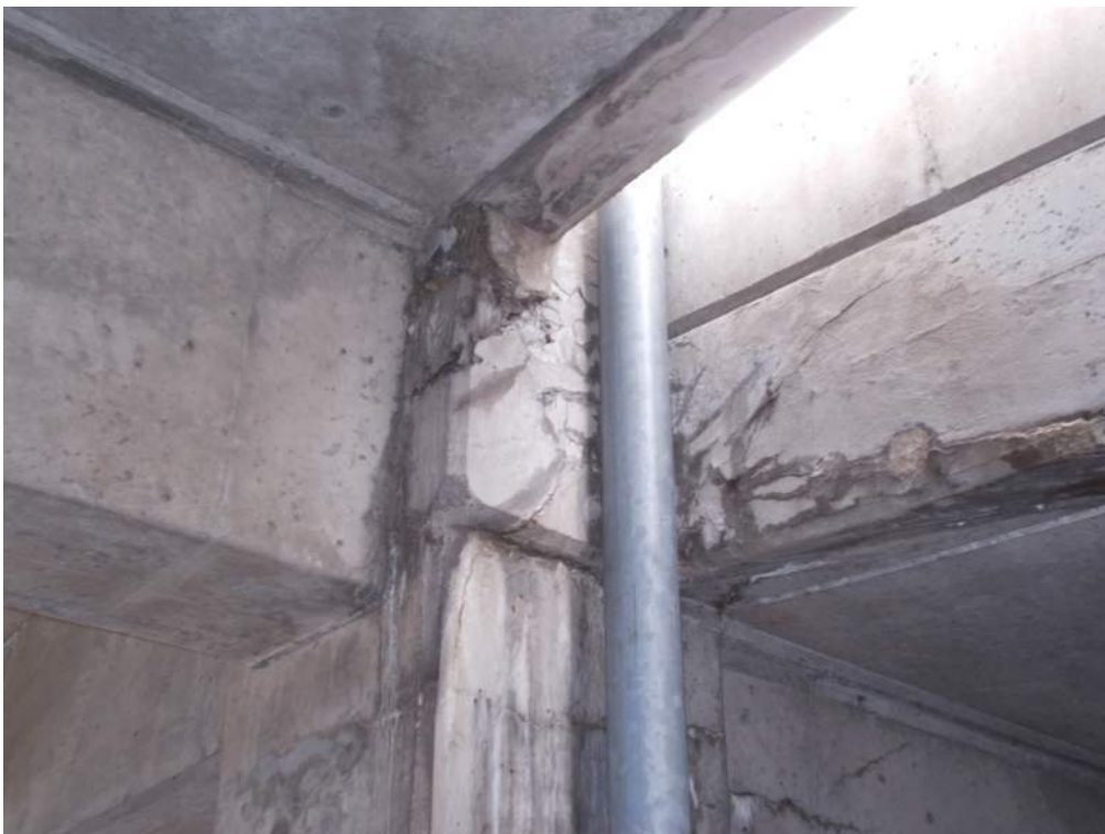
Photo 6 – Original Structure – Crack and spalled concrete in column at Grid E/4
