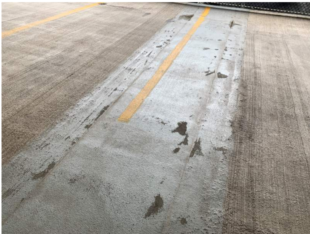
Photo 8 – Expansion Structure – Failed traffic coating over pour strip
